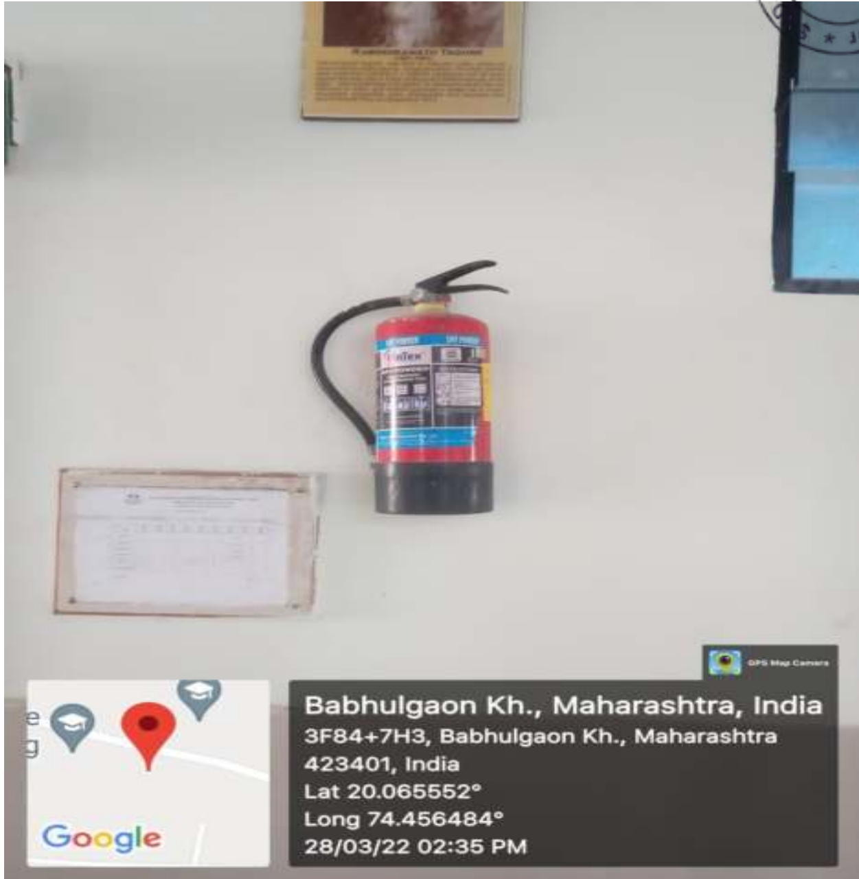
PHOTOS OF FIRE EXTINGUISHER INSTALLED IN THE CAMPUS
